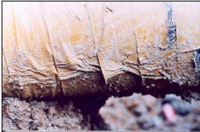
SOIL STRESS FAILURE
