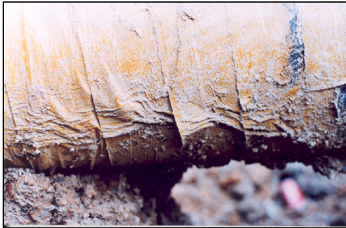
SOIL STRESS FAILURE
