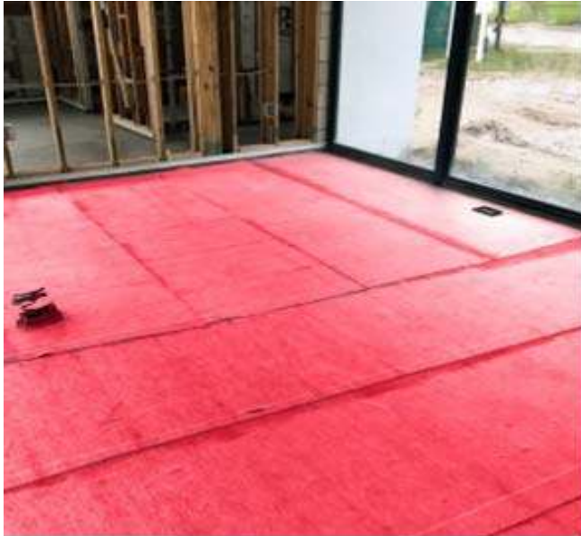
TERM Tile Underlayment Barrier installed in The New American Home – 2017 , built by NAHB in Orlando, FL
