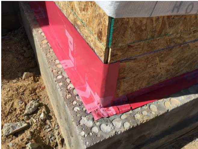
Above left is TERM Flashing Barrier installed on a residence in Waco, TX. Above right side of the corner is shown the previously installed TERM Sil Plate Barrier tie-in to flashing
