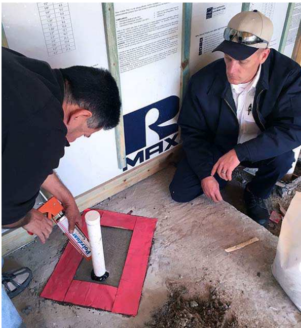
TERM All Pest Bath Trap Barrier being installed in The New American Home 2017 , an NAHB concept home to be introduced at the January 2017 International Builders Show in Orlando, FL
