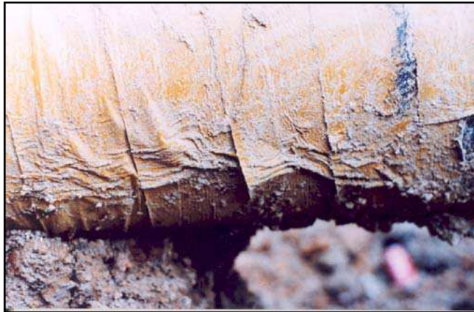
SOIL STRESS FAILURE
